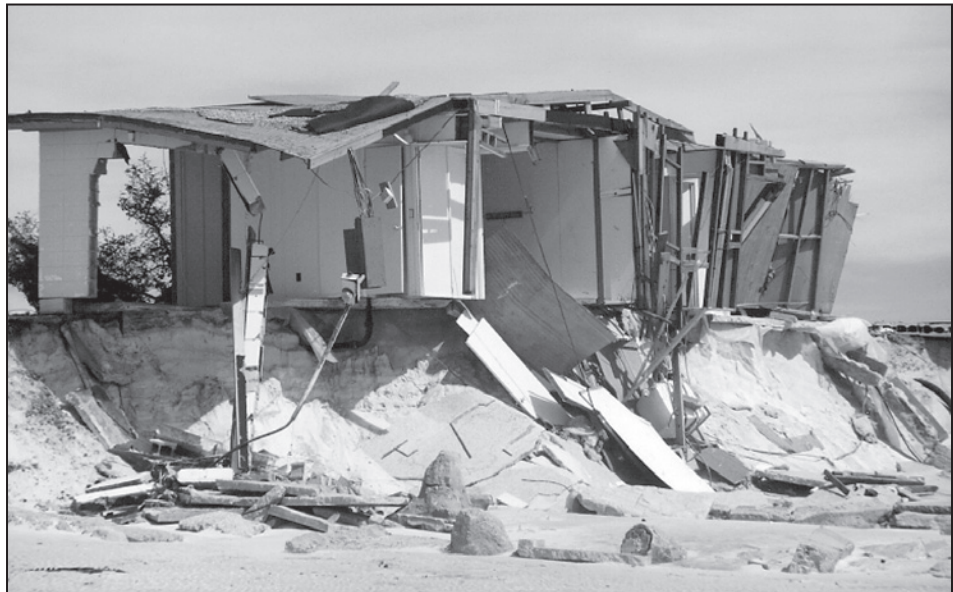
Figure 3-8. Large, fast-moving waves combined with erosion and scour to destroy this Gulf of Mexico home during Hurricane Opal
